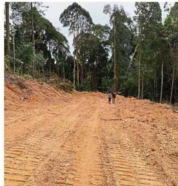
Land clearing works going on at a portion of the land in Bukit Cerakah for a residential project, which has been approved by the authorities.
